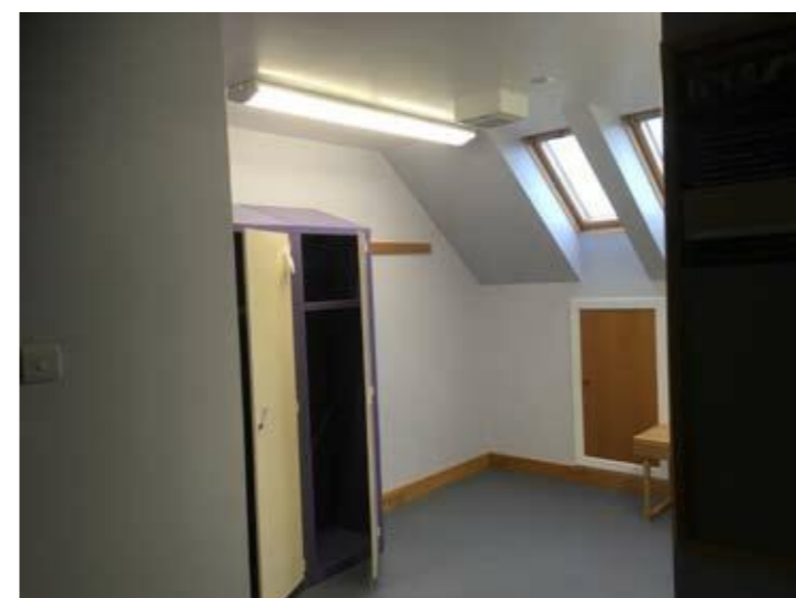
Potential bedroom (note high windows & escape issue)
