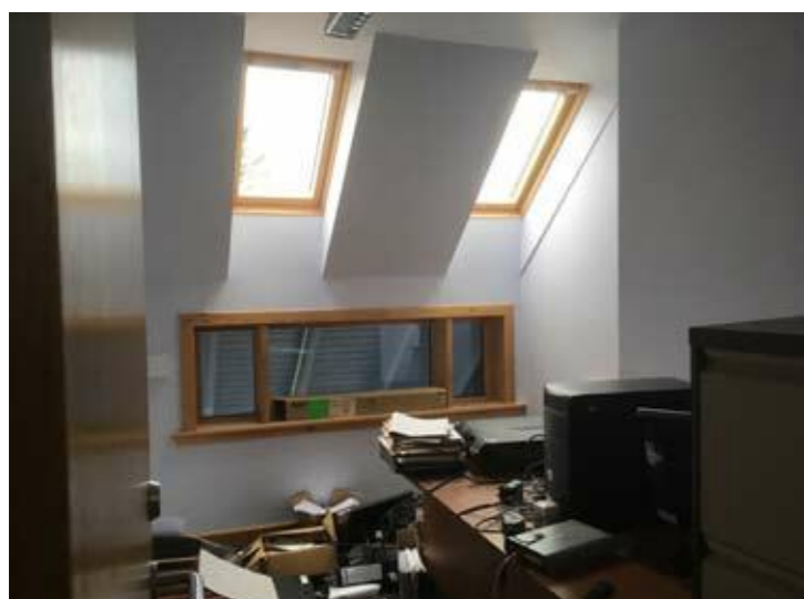
Potential bedroom (note high windows & escape issue)
